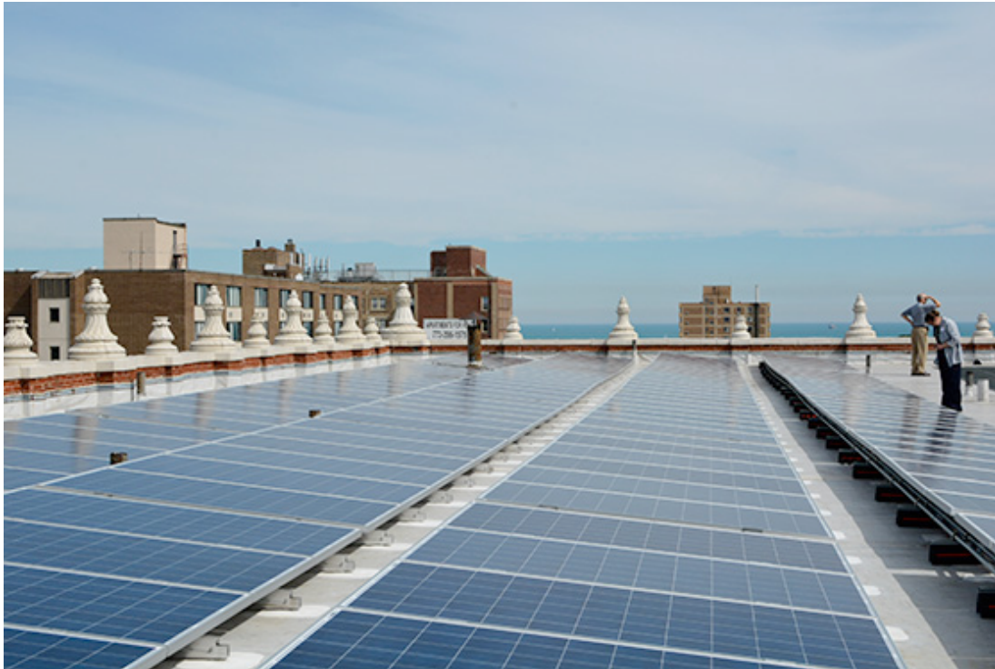
Solar Panels on top of ICA GreenRise Building Photo credit: Seva Gandhi
